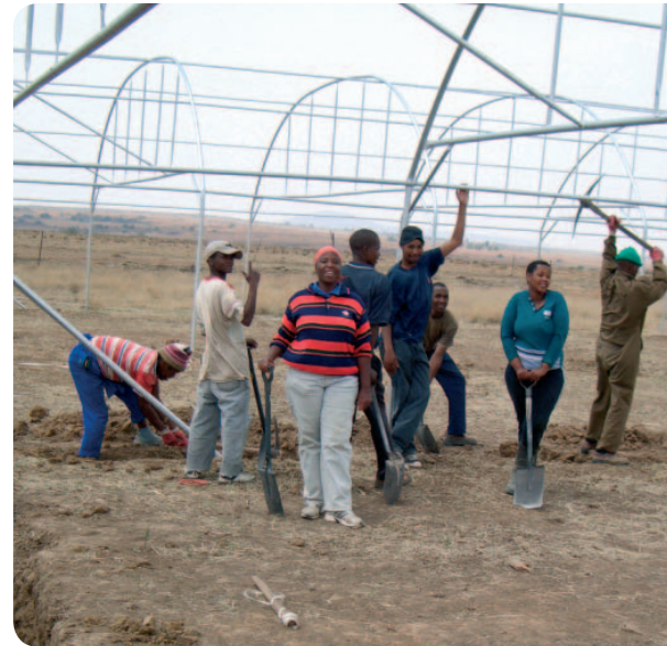
Members of the Blackthorn hydroponics project in the process of erecting one of the six tunnels.
