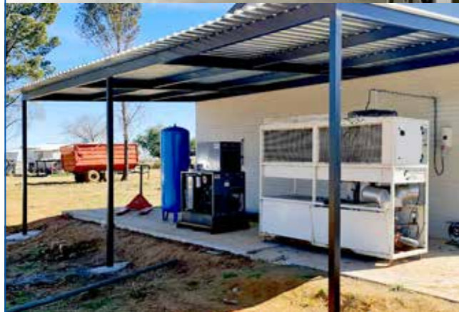
Glycol chilling plant and compressor installed on outside of the building
