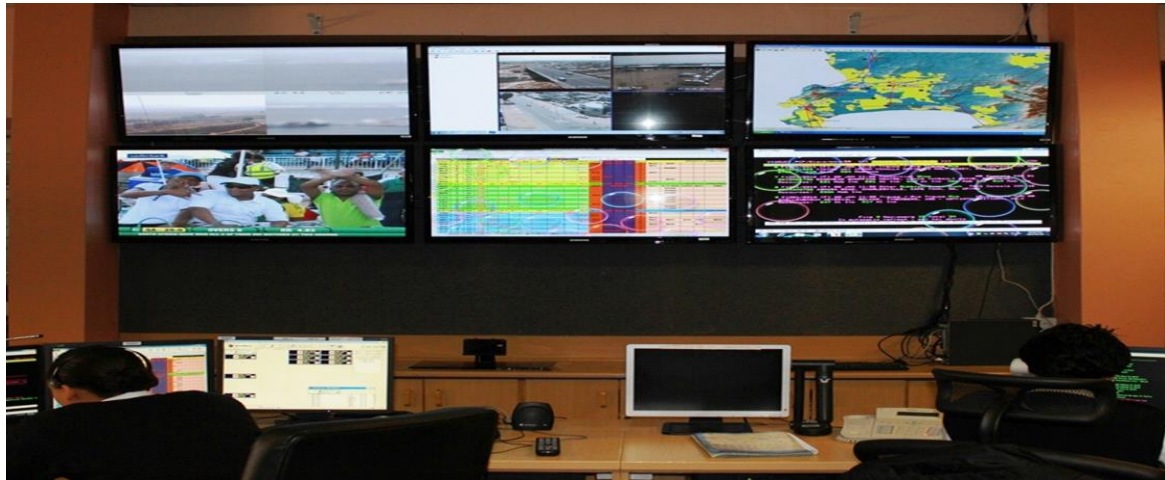
Figure 2.14: Command and control centre Source: Everts (2014)
