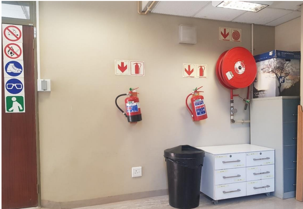
Figure 4.9 Fire extinguishers located at the chemical laboratory
