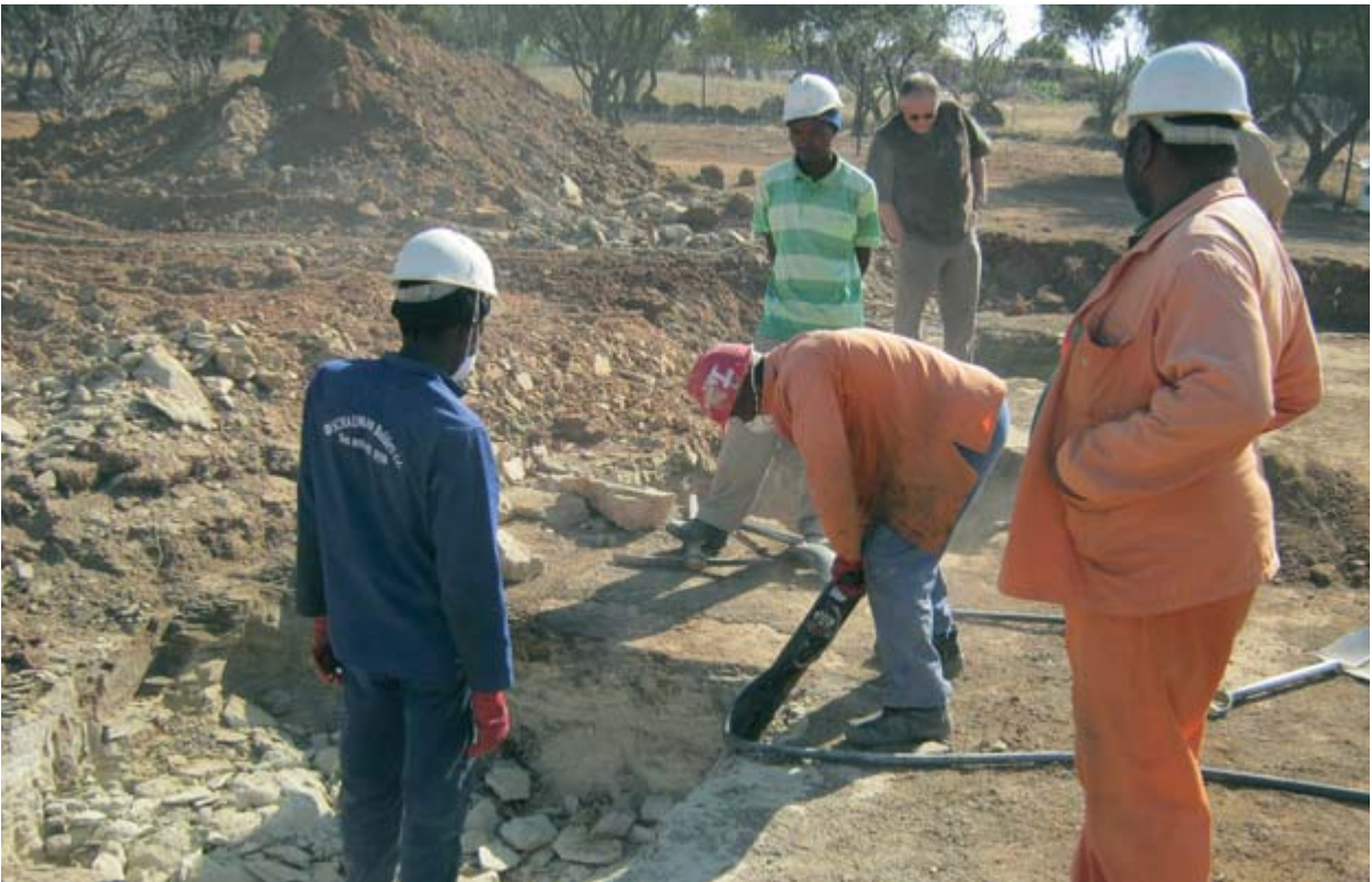
Excavations for the Department's new core storage facility. Prof W van der Westhuizen can be seen inspecting the excavations (middle, back).
