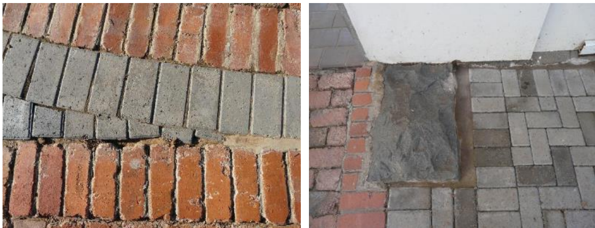
Figure 16: Bricks cut into unfeasibly small segments resulting in a poor junction (left) and a seemingly random stone incorporated at the base of a column.
