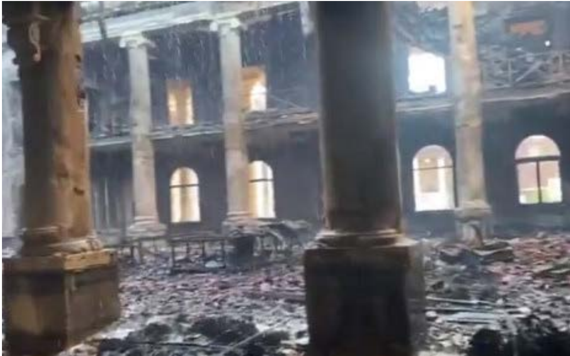
Figure 1: African Studies Collection after the fire incident on 18 April 2021. Photo source: https://www.news.uct.ac.za/article/-2021-04-23-ucts-historic-jagger-reading-room-lost-to-fire
